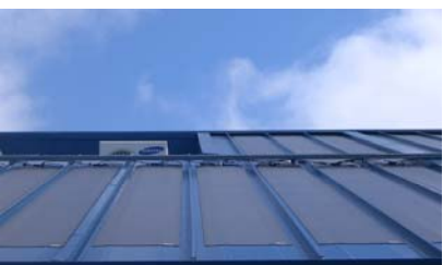
Bollinger Canyon School, 130KW PV System
