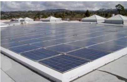
Doyle Library, SRJC, 60KW PV System
