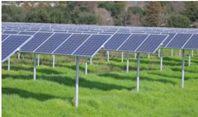
Napa Valley College, 1MW PV System
