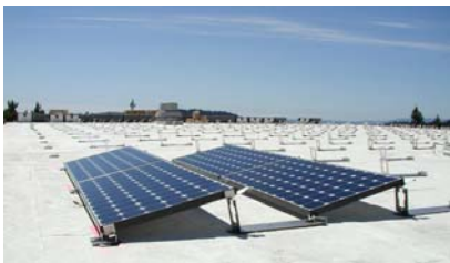
University of San Francisco, 500KW PV System
